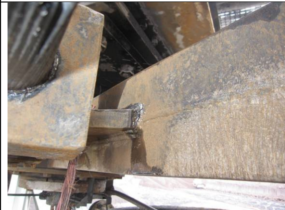
Photo #59 – crack at weld
