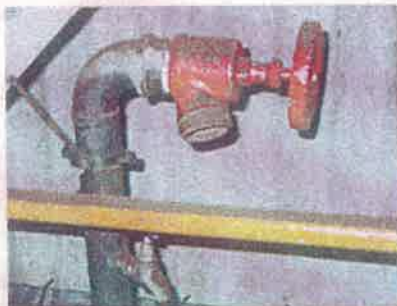
North Wall Hydrant
