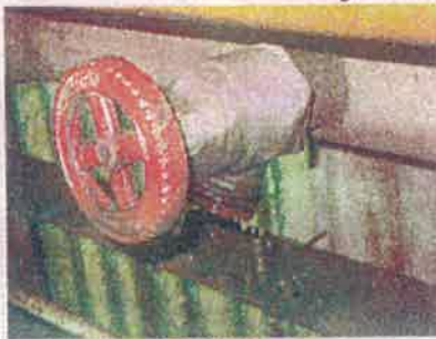
West Wall Hydrant
