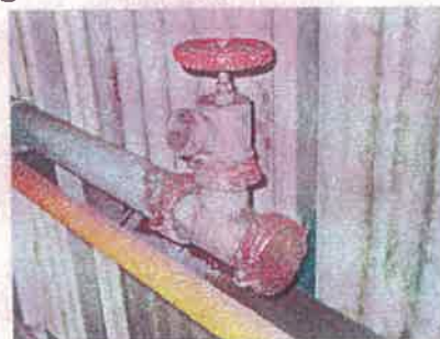
West Wall Hydrant
