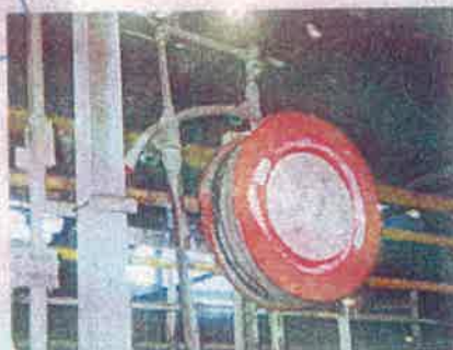
Control Room Walkway Hose Reel (HR-34)
