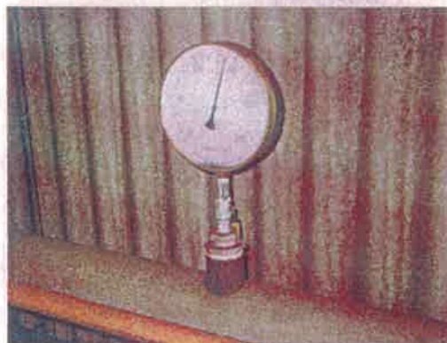
HSB West Wall GLBP Main Pressure Gauge
