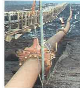
Looking Down The Length Of The Conveyor Valve Supplying Water To The 300mm F/Service Pipe, Hydrants & Sprays
