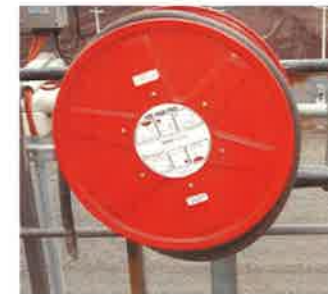
Fire Hose Reel
