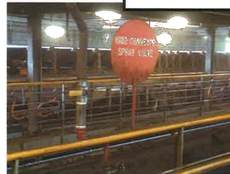
Valve spray lines located throughout the bunker
