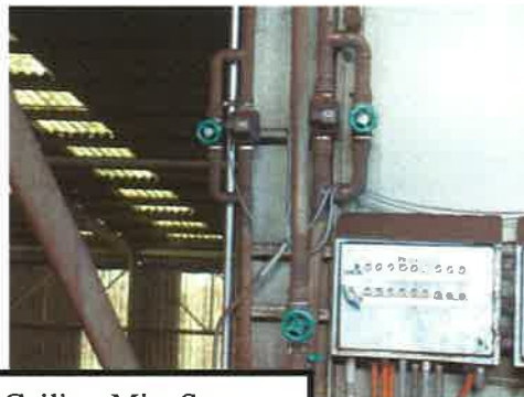
Bunker Ceiling Mist Sprays Located At North & South ends of Bunker
