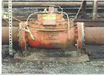
Typical Deluge valve Located At The Coal Face
