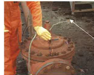
No Water Release from Drain pipe Valve Turning OFF
