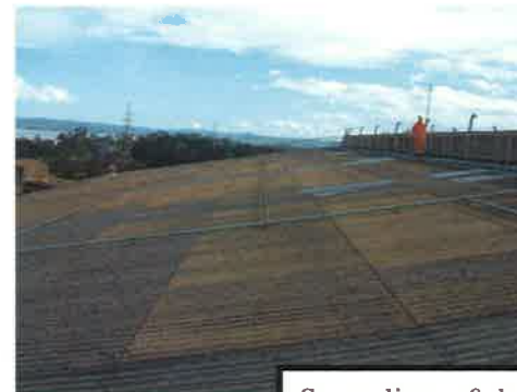
Spray lines & hydrants located on top of bunker roof line
