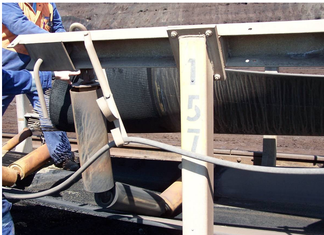
Idler Assembly 157 – CFA Fire Investigation Team
