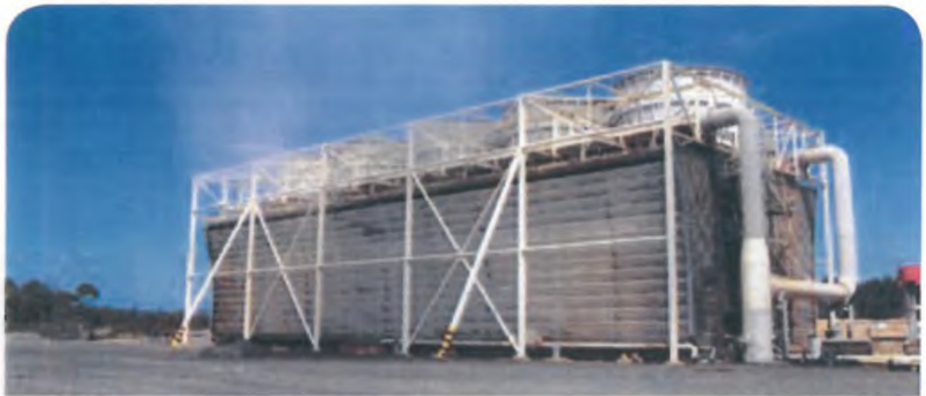
The Cooling Tower at Anglesea Power Station is one of the major sources of water usage.
