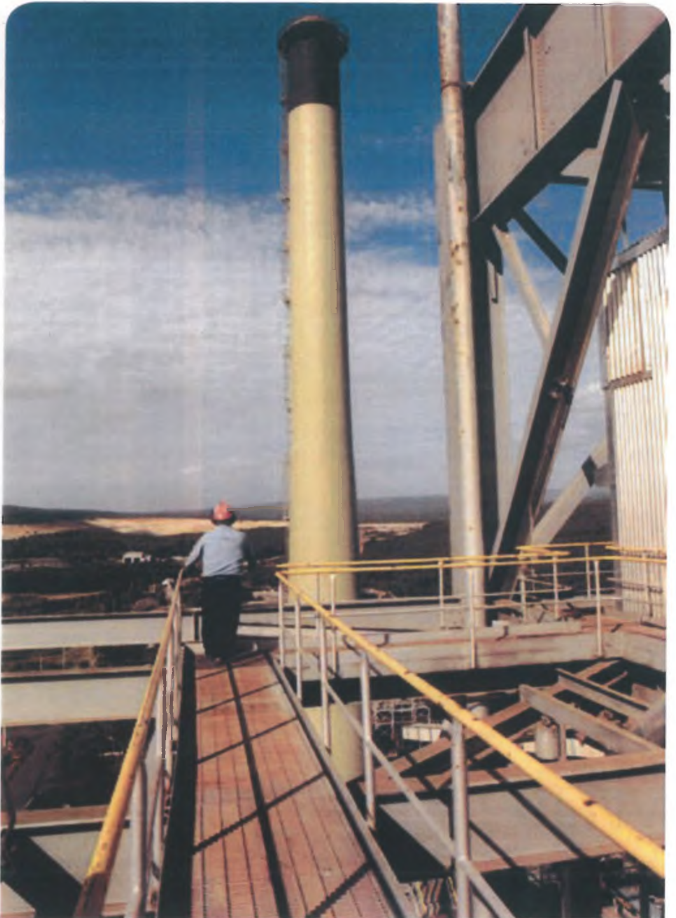
Management of sulphur dioxide emissions is currently Alcoa Anglesea's major environmental initiative.
