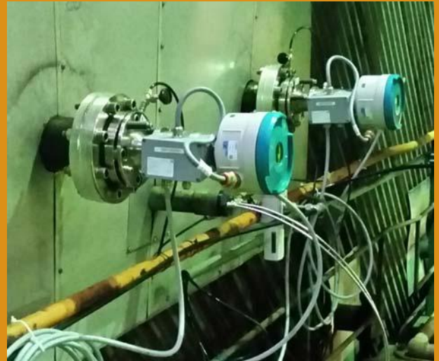
Oxygen and carbon monoxide lasers installed at Yallourn Power Station
