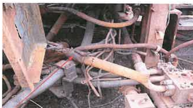
Damaged lead insulation connecting from engine to auto-shutdown box. System shorted on adjacent hydraulic hose metallic covering and ruptured the return hydraulic line.
