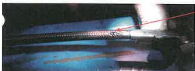
Hydraulic hose from turbocharger on haul truck ruptured by its heat shield cover. The incorrect placement of the shield caused continual abrasion of the outer metal hose sheath and fluid spray onto hot engine components.
