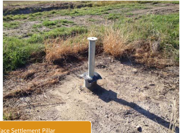
Surface Settlement Pillar
