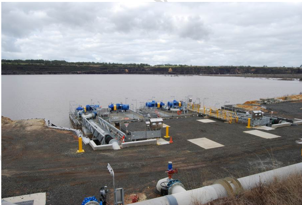
Figure 21 - Fire Service Pond Pumps
