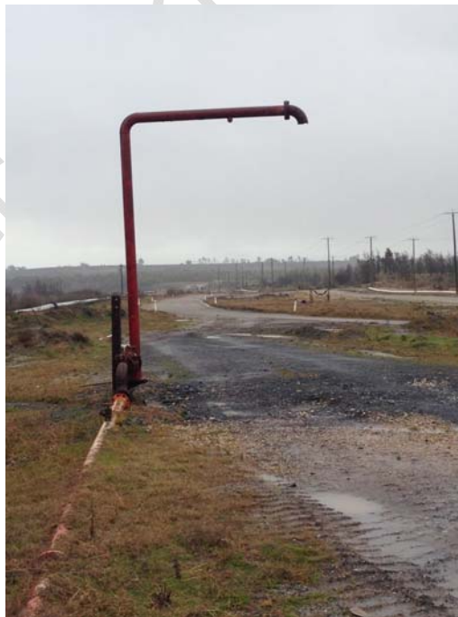
Figure 33 - Typical Tanker Filling Point
