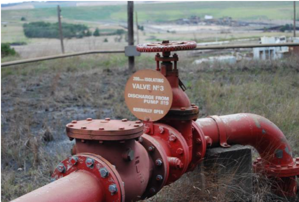
Figure 32 - Fire Service Infrastructure Labelling
