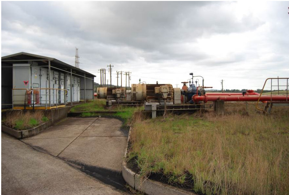
Figure 26 - RCB Booster Pumps
