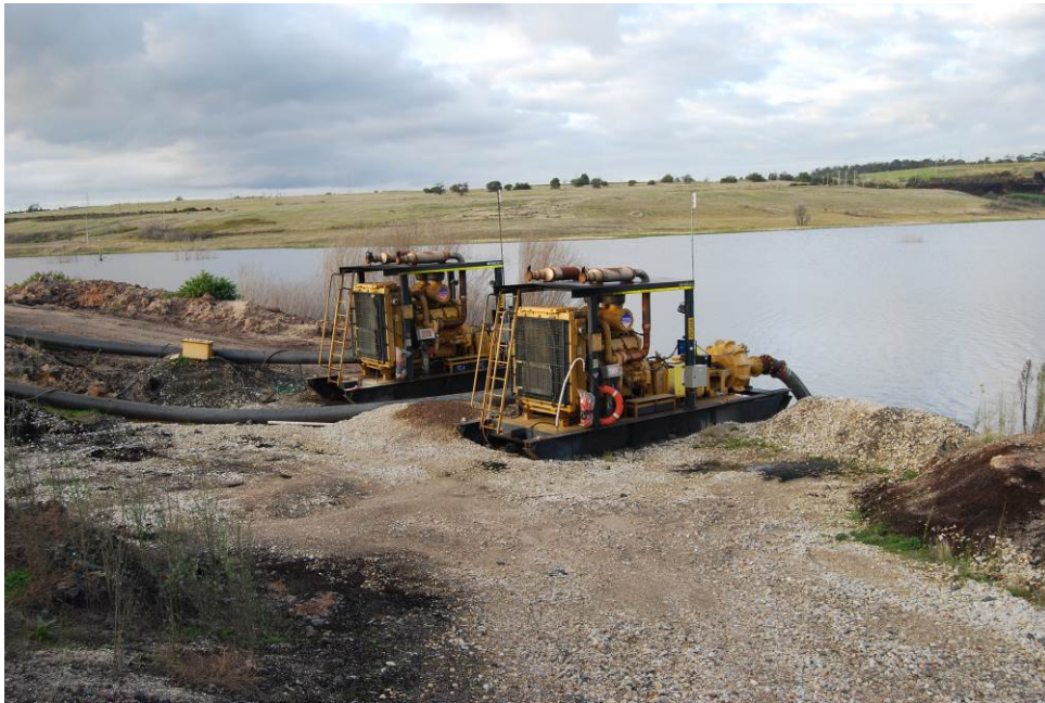
Figure 20 - Fire Service Pond - Emergency Diesel Pumps
