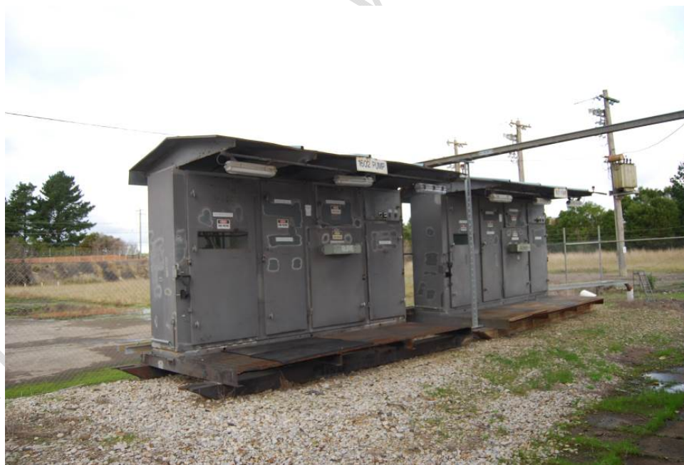
Figure 23 - Latrobe River Pumps - Electrical Cubicles
