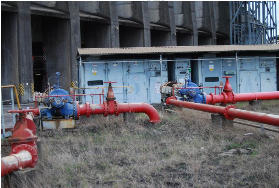
Figure 25 - RCB Booster Pumps
