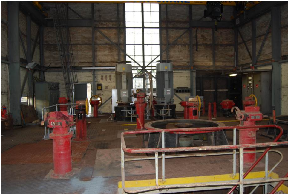
Figure 22 - Latrobe River Pumps - Nos 1601 and 1602
