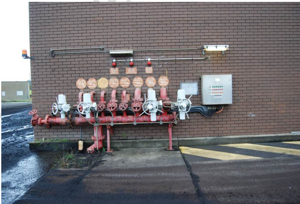
Figure 39 - RCB Fire Service Valve Station
